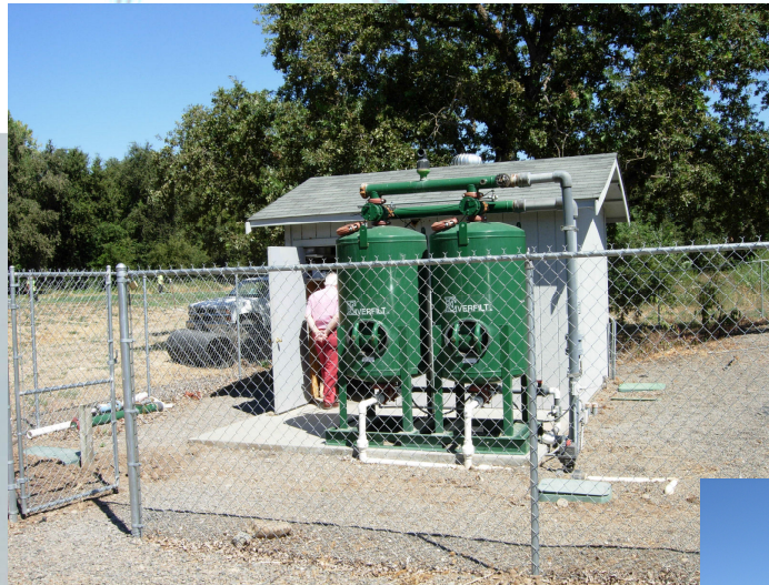
3,000 gpd Pacific Campground
