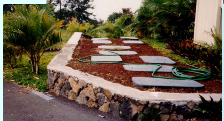
10,000 gpd-Captain Cook Apartments, HI
